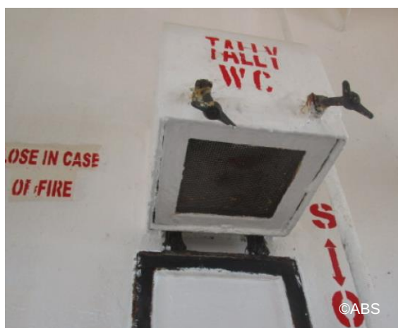
Ventilator dog broken/missing
