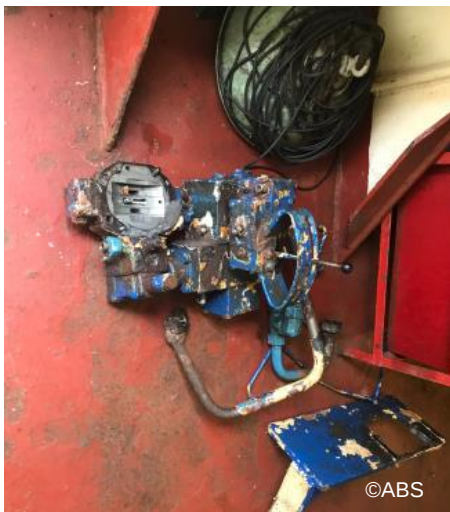
Damaged hydraulic motor for mooring winch removed
