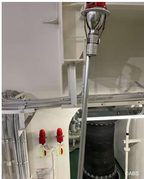
Testing engine room fire detector after repair
