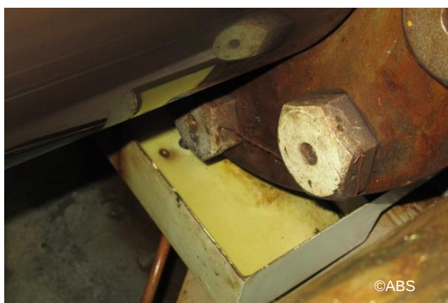
Steering gear leaking oil
