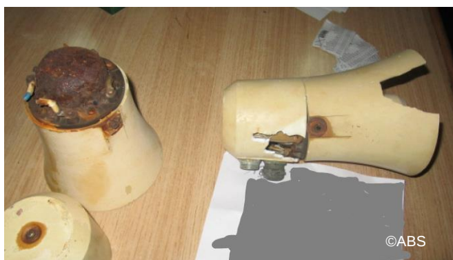
Public address system speakers damaged
