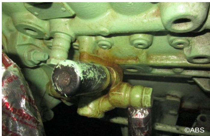
Emergency diesel generator high pressure pipe leak
