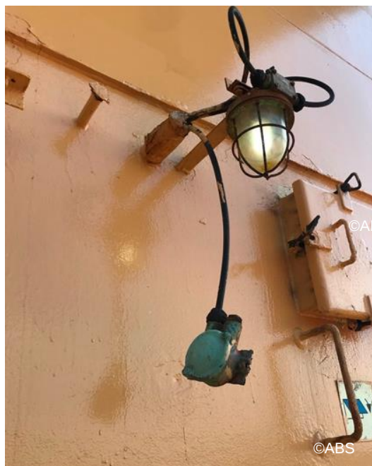
Damage to electrical installations
