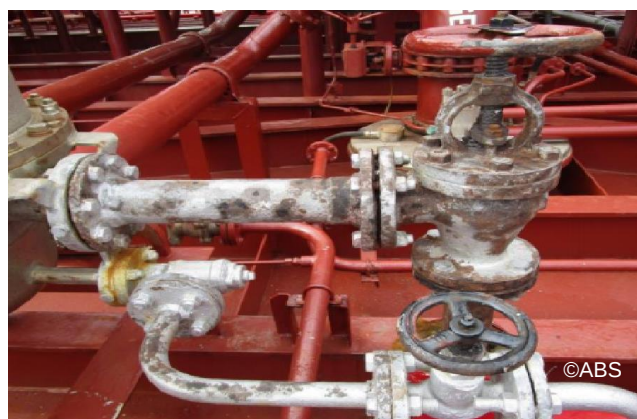
Steam pipe found with corrosion
