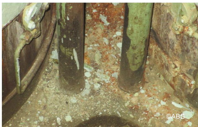
Main engine cylinder cooling water leak
