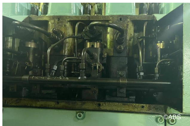
Main engine fuel pump leak
