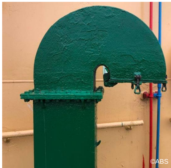
Ventilator found corroded – after
