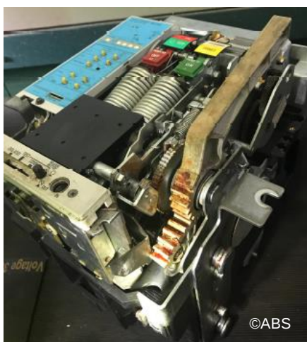
Emergency switchboard air circuit breaker damaged
